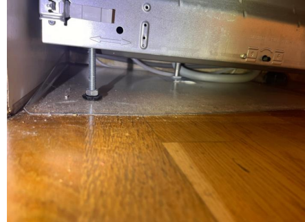
Plastplate under oppvaskmaskin
