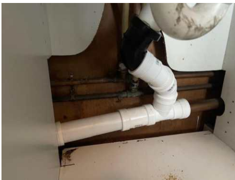
Røropplegg under vask
