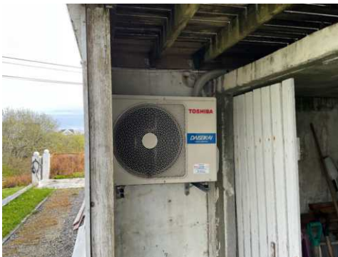
Varmepumpeaggregat under altan.
