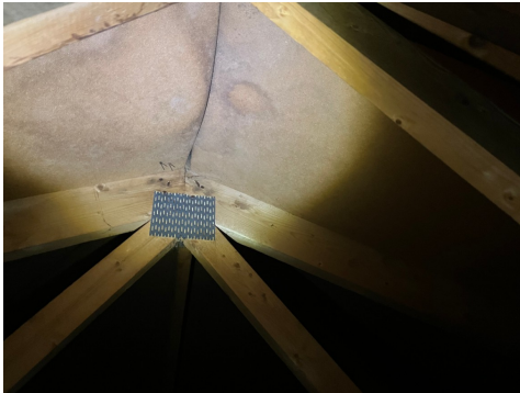
Fuktmerker i undertaket.
