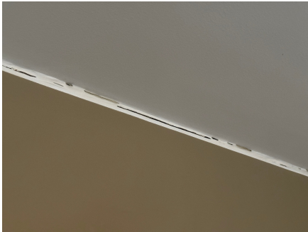
Sprekker i fugemasse overgang tak/vegg
