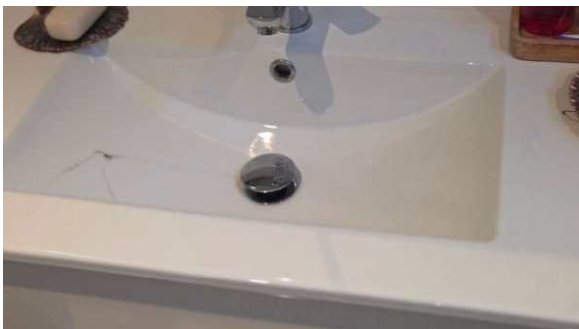
Sprekk i servant
