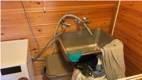
Opplegg for vaskemaskin
