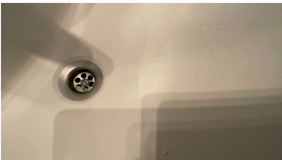
Riss/sprekk i servanten.
