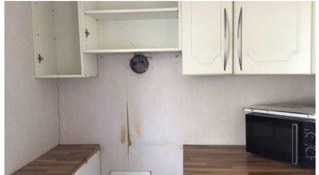
Hull for kjøkkenventilator.
