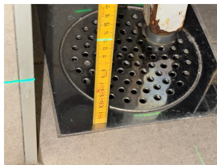
Fallforhold ca. 130 mm topp slukrist
